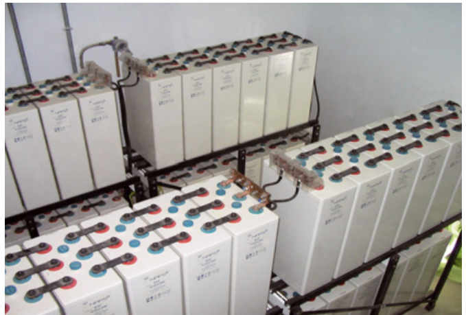
Solar photovoltaic industrial system
